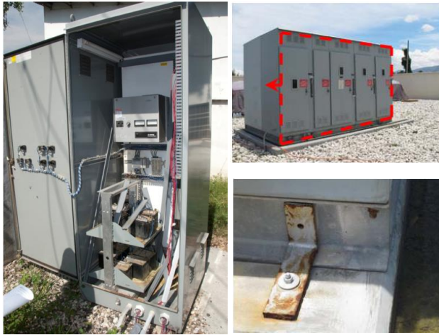
(a) General electric cabinet in Haiti earthquake (Goodno et al. 2011)
